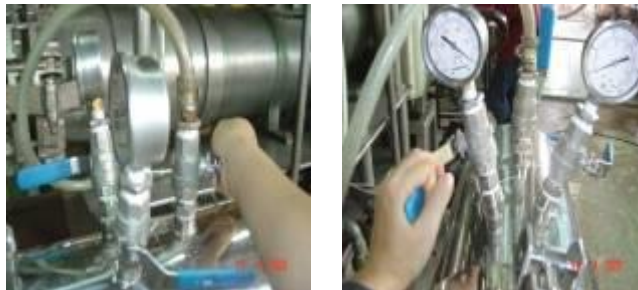
Figure 4. Open valve of pressurized tank (left), open gauge vacuum valve (right).
